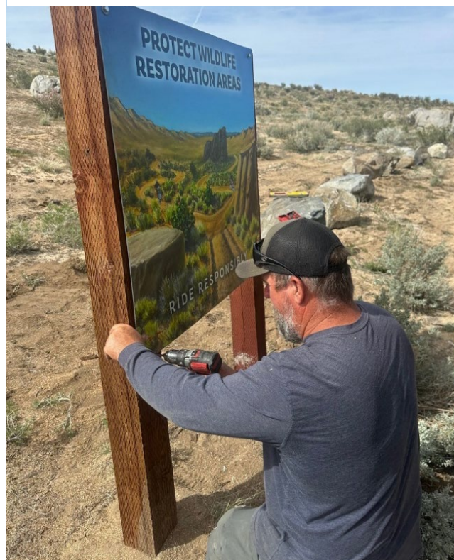
Figure 3 - Eagle Lake OHV project includes the installation of signs at restoration site.
