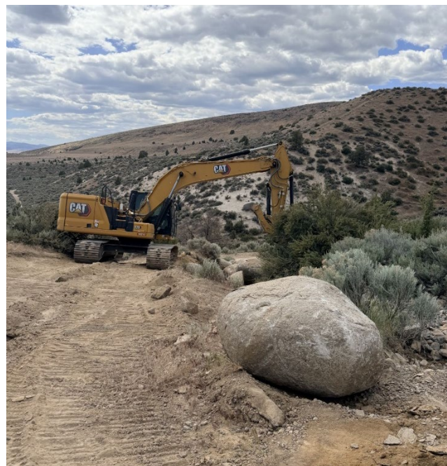
Figure 2 - Eagle Lake OHV projects use an excavator to place boulders and complete trail work.
